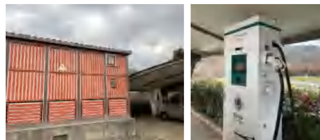
Figure 5-1-1-3 Charing and battery for electric cars
