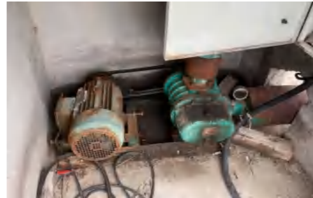
Figure 5-2-1-10 Oxygen supply equipment
